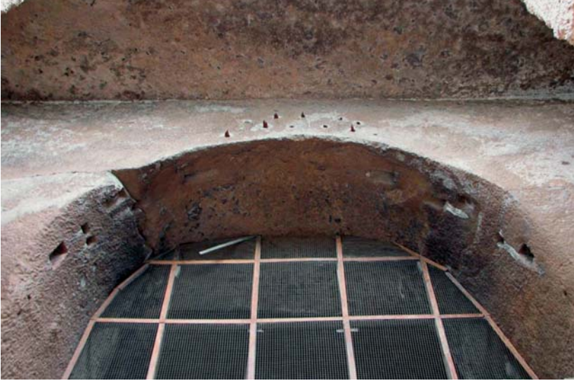
Fig. 27. View of the upper façade inside the veranda. Note the cracks, most visible on the left side of the caitya window, and the remains of wooden timbers projecting from mortises between window and ceiling. Cave 3 ( caitya hall), Kānherī, 1 st –2 nd century CE.
