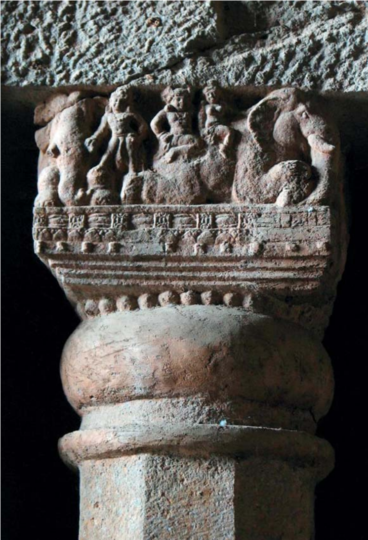
Fig. 22. Capital of the seventh pillar on the left side of the hall. Note the crack intersecting the head of the elephant on the left corner and proceeding diagonally above the capital. Cave 3 ( caitya hall), Kānherī, 1 st –2 nd century CE.
