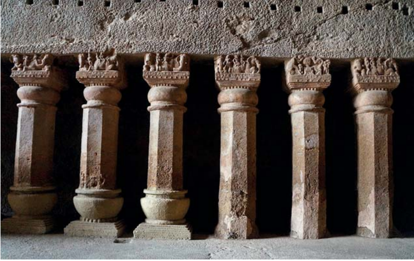
Fig. 21. Fourth through ninth pillars on the left side of the hall, with crack traversing diagonally from the vaulting (upper right of photograph). The bases of the fourth, fifth, and sixth pillars display recent attempts at restoration in this photograph. Cave 3 ( caitya hall), Kānherī, 1 st –2 nd century CE.
