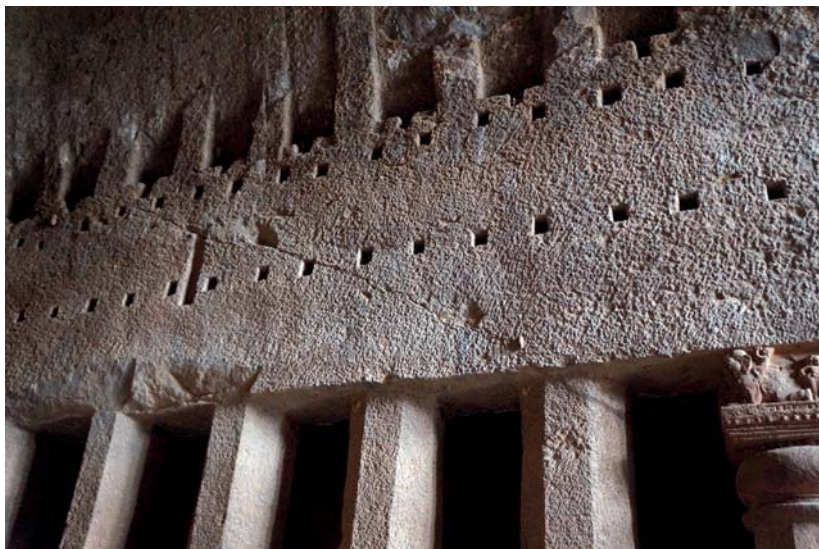
Fig. 20. Right side of the hall with crack extending diagonally from the vaulting and intersecting the unadorned seventh pillar (partly filled in with cement but still visible). Note also the cavity or depression above the ninth, tenth and eleventh pillars present on the left side of the photograph. Cave 3 ( caitya hall), Kānherī, 1 st –2 nd century CE.
